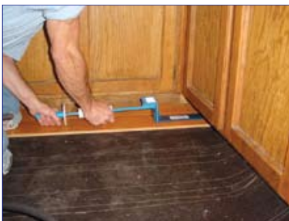
Lam-Hammer with the extension attached, to get under a cabinet toe kick.
